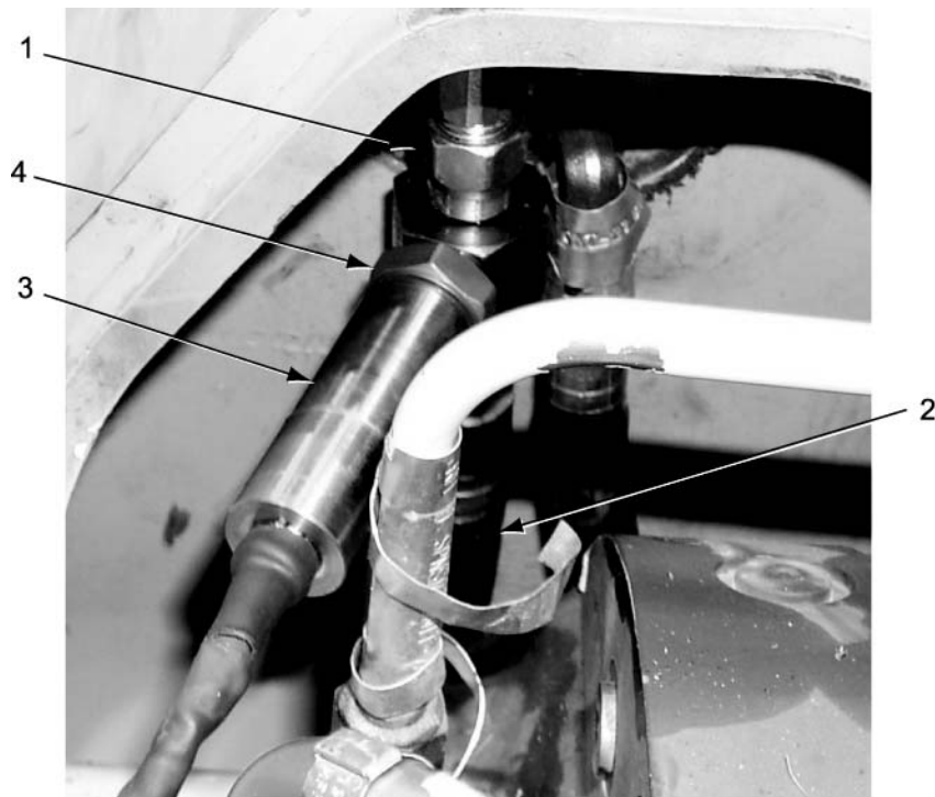
Figure 3-46. Installation of Right Side Bump Stop Cylinder Pressure Transducer T8
